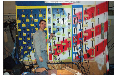
Figure 7.12 So many camera triax cables converge on the truck compound for the Super Bowl that the setup crew uses a wooden board to terminate each cable. The cables are statically tested (without the actual cameras connected) and then a short piece of triax is run from this board to one of the four trucks that support this large platoon of cameras. This setup makes it easier to troubleshoot problems, and to find and quickly use any of the numerous spare cables as backup. Notice that each cutout and slot holding the end of a triax cable is labeled as to the location of its other end. The crew refers to this board as “the chrome cow.” (Source: Marty Elbeck - NEP)
